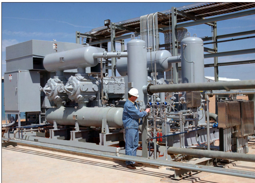
Model JGZ/4 in Snyder, Texas, being used for carbon dioxide injection.
